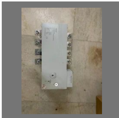
Axon ATS Automatic transfer switch
